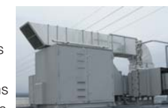
Equipment for the treatment of EOG emissions
