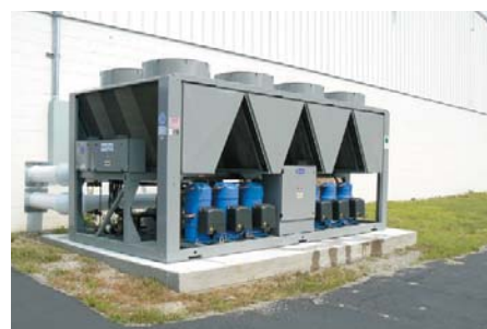
High-efficiency water-cooling system
