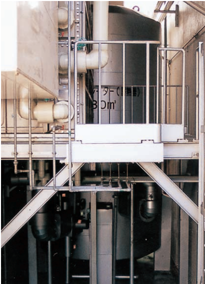
Steam accumulator at the Fujinomiya Factory (center back)
