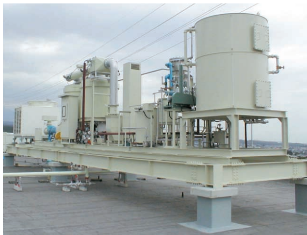
Dichloromethane recovery facility (Ashitaka Factory)
